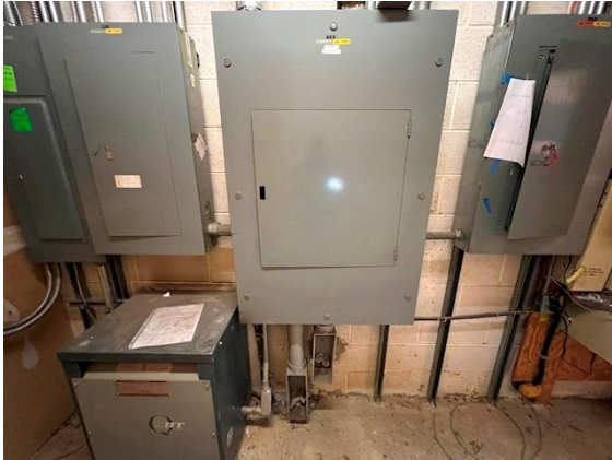
Electrical: Main electrical service in utility room
