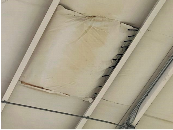
Roof Insulation: Evidence of past leak
