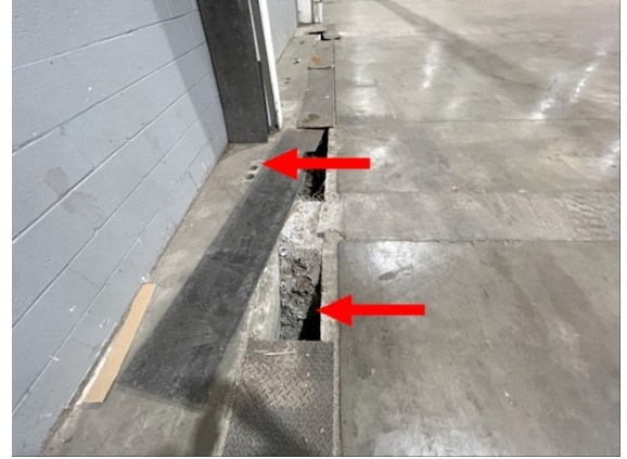
Floor / Slab: Buried conduit and access plates
