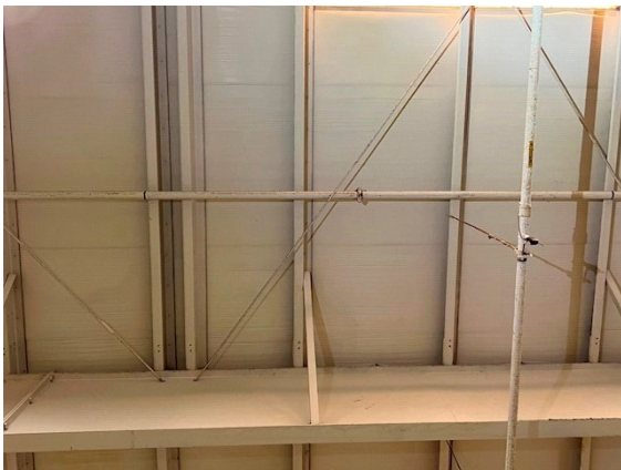
Roof Insulation: Most of the roof insulation panels appeared to be in good condition
