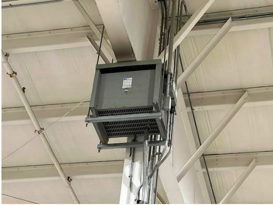
Electrical: Transformer mounted in ceiling of warehouse
