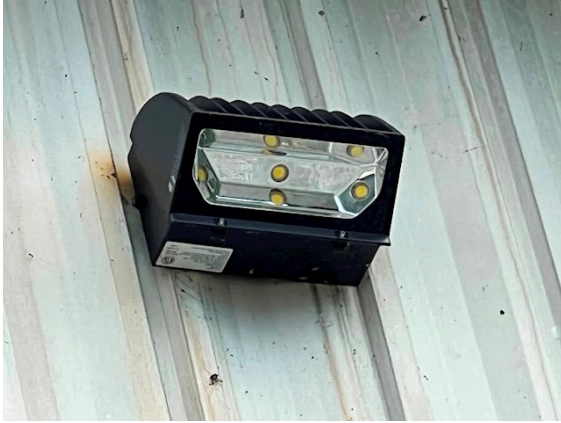
Exterior Surface: Wall pack LED lighting
