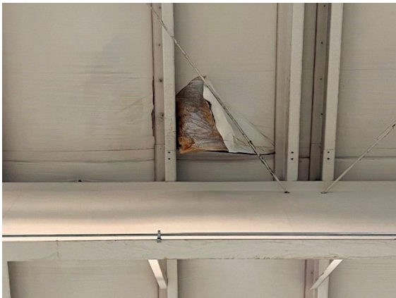
Roof Insulation: Evidence of active leak (northeastern quadrant of roof)
