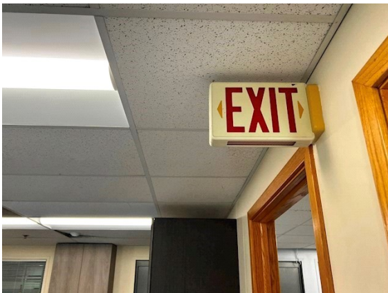
Life Safety: Exit sign not working
