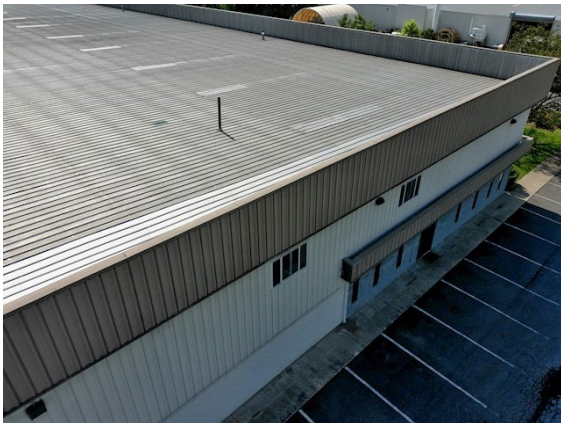
Roofing: Overview picture of parapet wall on west and southern perimeter of roof
