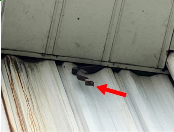
Parapet Wall System: Weather seals hanging down in some locations
