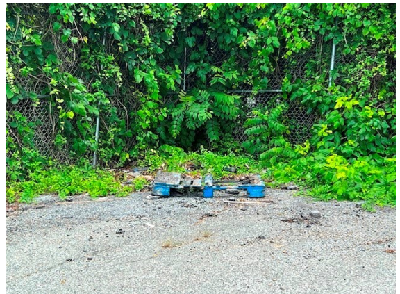
Fences / Enclosures: Vegetation growth should be removed from fencing
