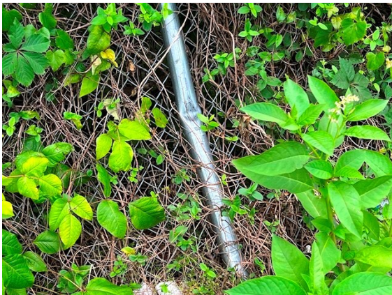
Fences / Enclosures: Fence pole on east side of yard bent and fence leaning in this area
