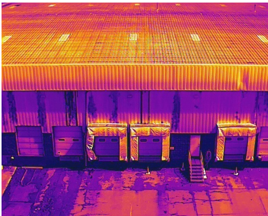
Parapet Wall System: Infrared image of south side showing evidence of gutter leaks
