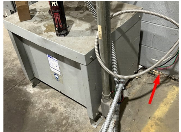
Electrical: Transformer to the right of drive in door on west side (note exposed wiring)
