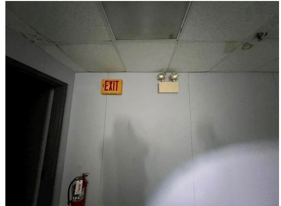
Life Safety: Exit signs did not work or test properly
