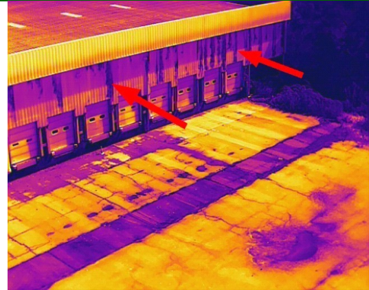
Parapet Wall System: Infrared image of south side showing evidence of gutter leaks
