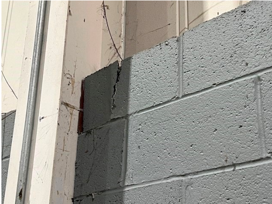
Interior Foundation: Top edge block cracked near northeastern corner of building along back (east) wall
