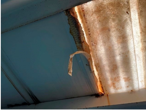
Roof & Interior Structure: Insulation tape peeling away from water intrusion
