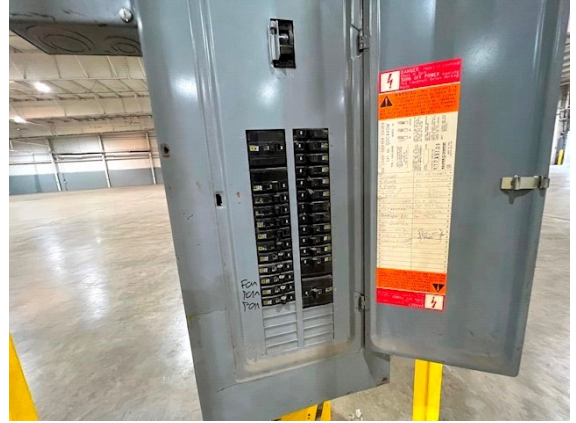
Electrical: Panel for ceiling mounted transformer
