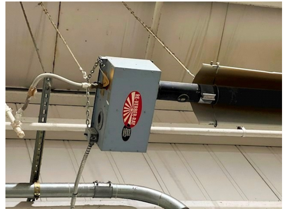
Warehouse Heating: Burner unit
