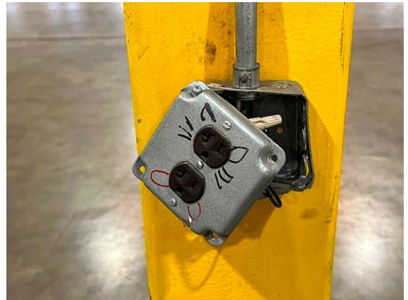
Electrical: Outlet cover not secure
