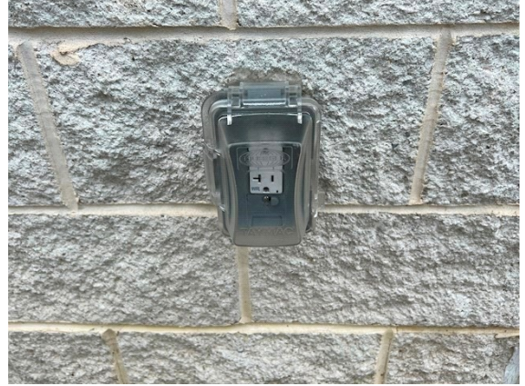
Exterior Surface: Exterior GFCI protected and covered outlets
