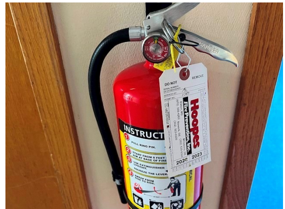
Life Safety: Fire extinguishers had a current inspection tag and good for use
