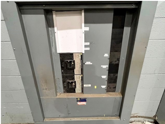
Electrical: High voltage panel in warehouse
