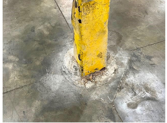
Roof & Interior Structure: Dented steel column with concrete repair evident
