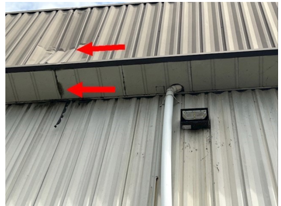
Parapet Wall System: Damage to parapet wall and evidence of gutter leaks
