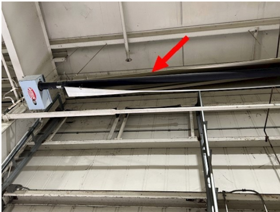
Warehouse Heating: Twisted heat shield
