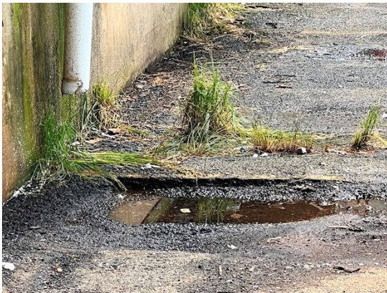
Grading / Drainage: Ponding observed in some low lying areas in the dock/loading area
