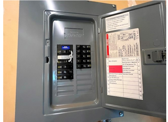
Electrical: Appears to have had a backup generator installed at some point
