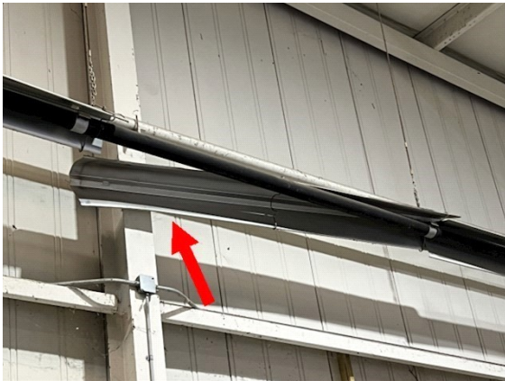
Warehouse Heating: Displaced heat shield
