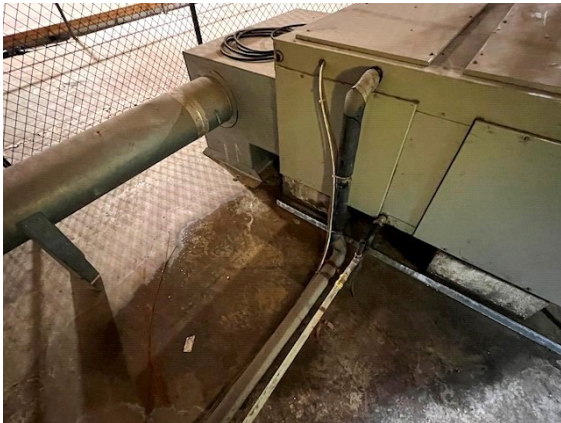
HVAC: Liquid line and primary condensate line
