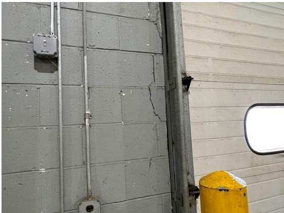
Interior Foundation: Vertical cracking observed to the left of freight door #3
