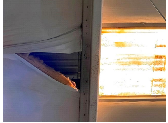
Roof Insulation: Evidence of past leak, dry on the day of inspection
