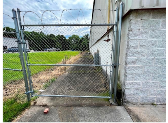
Fences / Enclosures: Second gate at northwest corner of building, secured with lock
