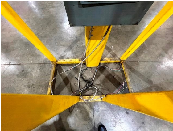
Electrical: Exposed wiring
