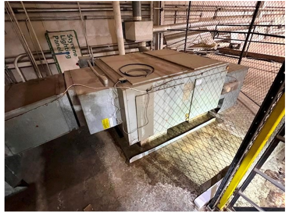
HVAC: Secondary condensate drain pan was full at time of inspection
