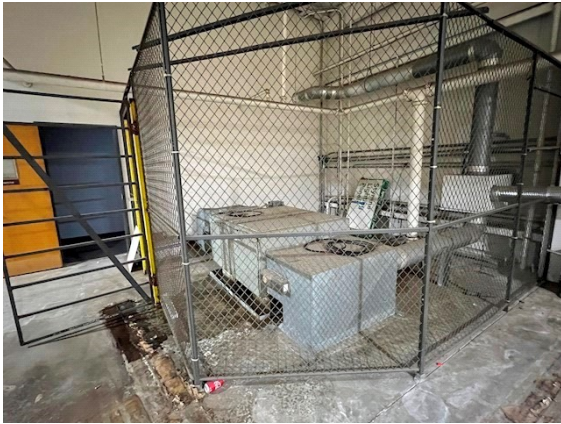
HVAC: Main air handler installed on 2nd floor mezzanine
